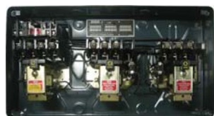
Interior View of MK1 SASD
