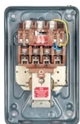
Interior View of MK2 DOL
