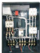
Interior View of MU-G30W FASD
