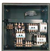
Interior View of MU-G20W FASD
